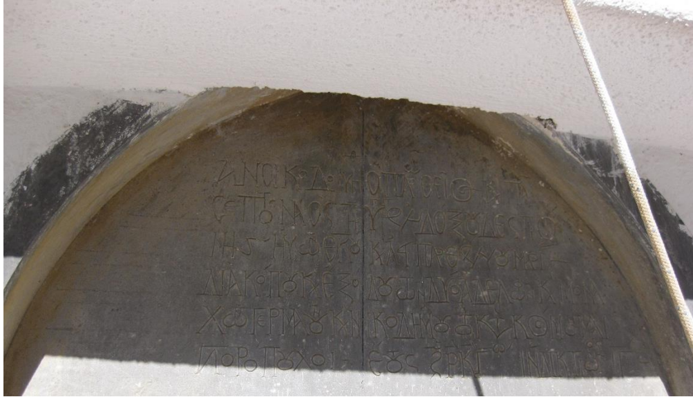
IMG_6119 The inscription over the door of the Panagia at Chamilo, showing how a recent crudely placed concrete block has covered the top of the arch (as well as shading the inscription!)
