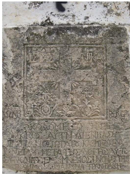
IMG_0364 Inscription on eastern bridge (on left side of parapet, on road side; dated 1852)
